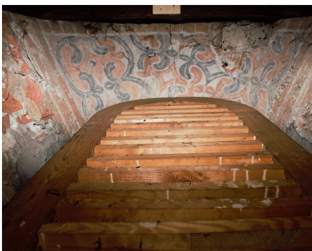
11. Zone above the Rosary Chapel, polychromies in the archway of the bricked-up presbytery window (photo by J. Kamińska, 2022)
