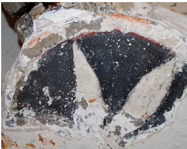
The probe on the bolt of the cross vault in the former sanctuary. The motif of a white solar rosette on the black background is visible on the primary layer of polychrome. The raised bordure is outlined with red iron pigment.
