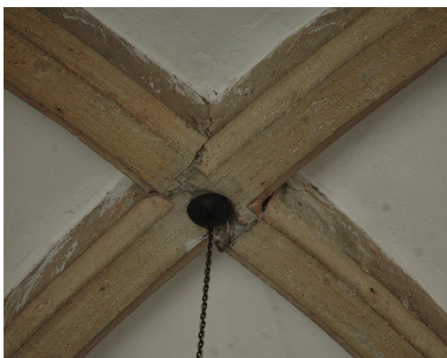
15. Ribs of the cross vault on the ground floor of the western tower (photo by author, 2014)
