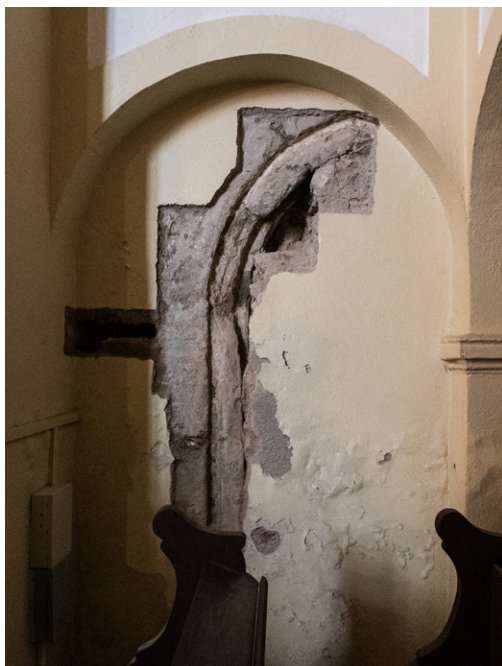
The north wall of the former sanctuary; the find of the stone lining of the Gothic portal
