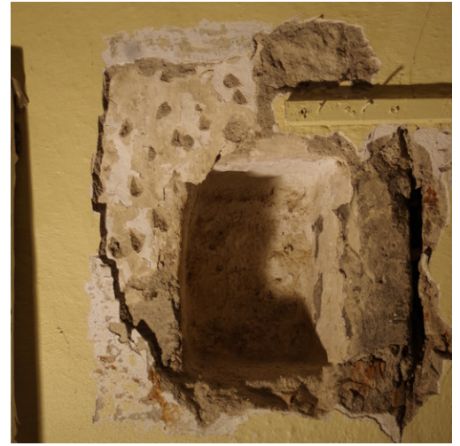
The niche on the south wall of the former sanctuary exposed in the probe; the architectural element is carved into a single stone monolith
