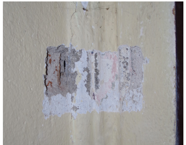
The probe on the lining of the south entrance to the nave in the narthex; the worked stone element of the Gothic portal is visible beneath layers of secondary surfaces
