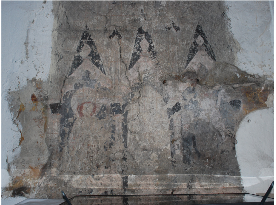
27. Wall-painting belonging to the south side altar in the nave of the church of Spišská Belá (photo by author, 2021)
