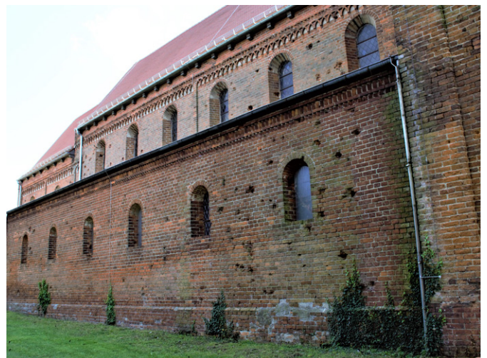
16. Northern façade of the parish church in Sandau (photo by J. Kamińska, 2021)
