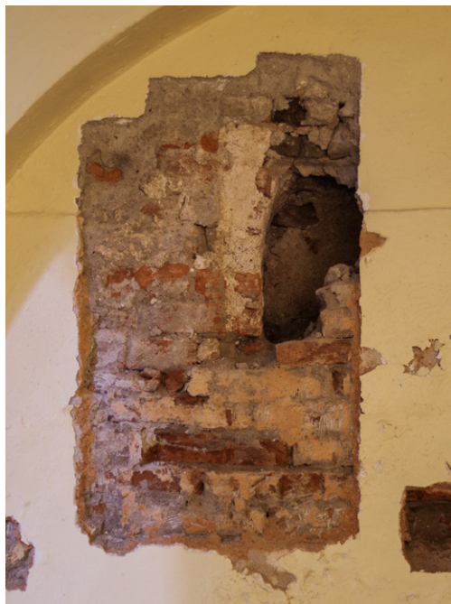
Part of the exposed niche (pastophorion) on the northern wall of the former sanctuary; the opening is made primarily of burnt brick
