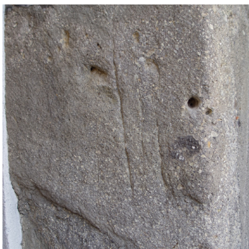
Detail of the right lining of the western portal; the so-called magic pits are visible in the mass
